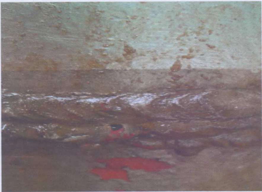
Picture showing pinhole on the wellhead.
